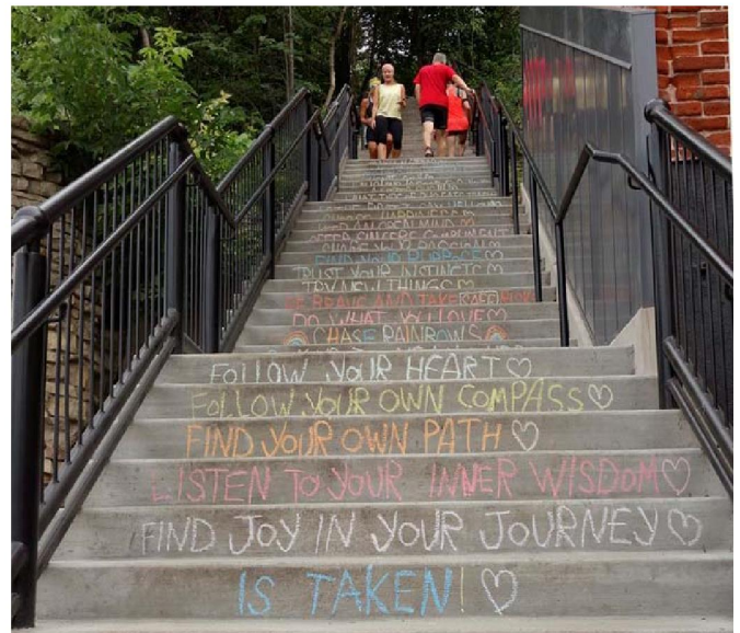
Public stairway reconstruction accompanied the adaptive reuse of the Joseph Wolf Brewery, 2018.
