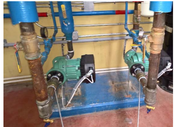
WWTP Boiler Pumps
