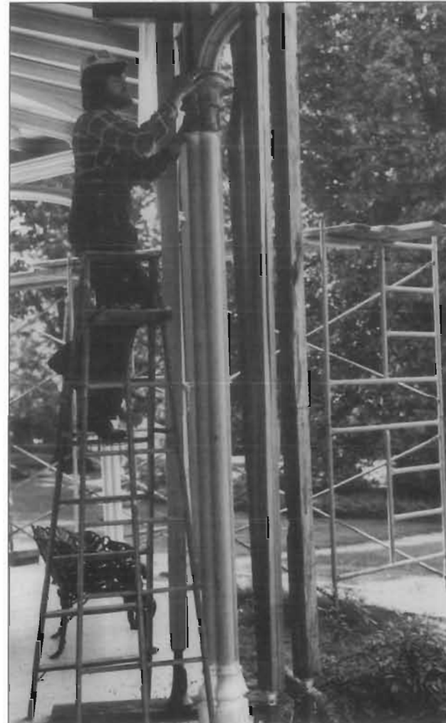
Careful inspection of porch features such as these column capitals is necessary before initiating a rehabilitation project.
