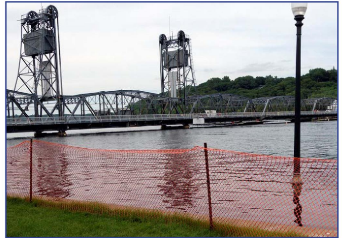
Stillwater Lift Bridge, 2018, during renovation as a pedestrian and bicycle path, and a foreground interpretive panel on bridge history and operation.
