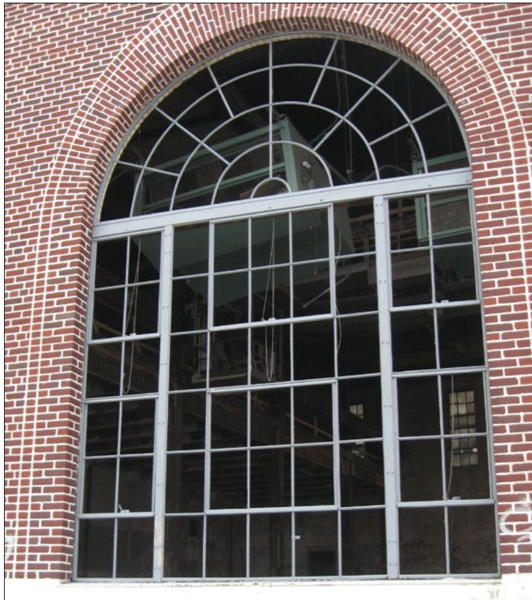
[12] This historic steel window has been cleaned, repaired, and primed in preparation for painting and reglazing.
