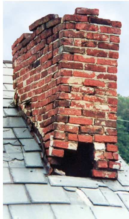
[7 a-b] This crumbling chimney was restored to its historic appearance using matching bricks.
