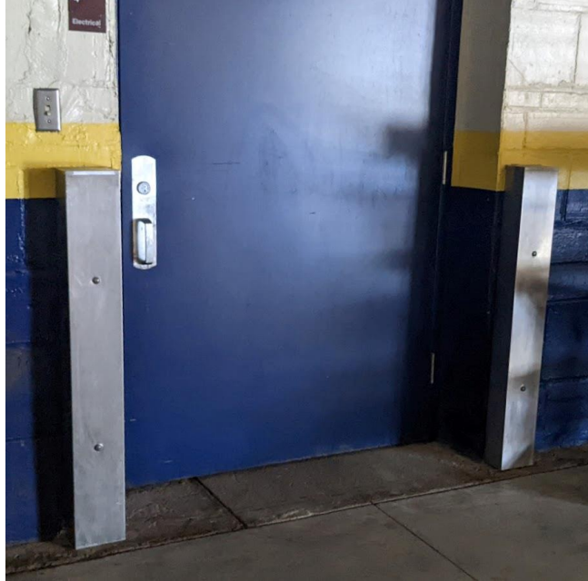
Figure 5-4 Stadium Electrical Room Flood Door with Posts for Stoplog Temporary Closure
