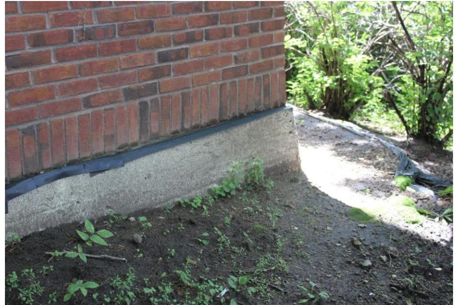
West slope eroding
