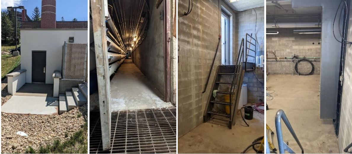
Figure 5-6 Pump House Door, Tunnel, Entrance Stairs, and Electrical Panel (left to right)
