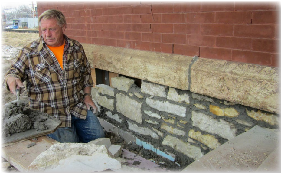
Stone mason applying the original foundation limestone cut by volunteers for facing on the new foundation
