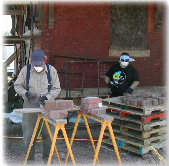
Volunteers cleaning mortar from bricks reclaimed from the old Washington school and donated by the City
