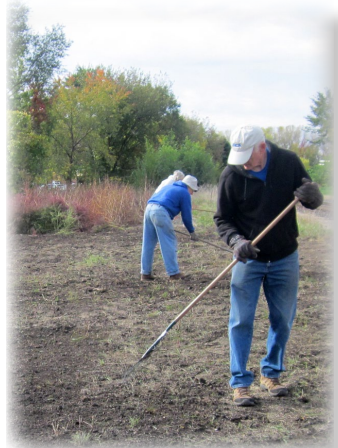
Volunteers raking and seeding the leveled area of the original depot site to fulfill the contract with railroad
