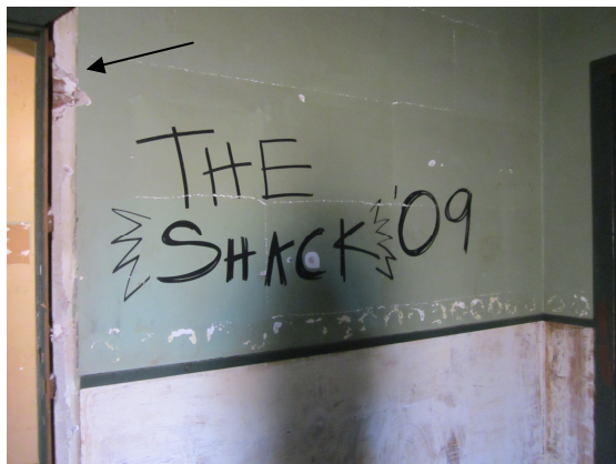
Walls: Plaster board and plaster added in 1944; plaster board cracked at seams during move (somewhat visible in above image). Arrow points to a hole we made in the 3/4" plaster which confirmed our suspicion that there was wood beneath.
