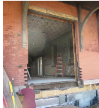
The large window opening was converted into an opening for the future double door that will serve as the handicapped accessible entrance. That entrance will be level with the pavilion floor.
