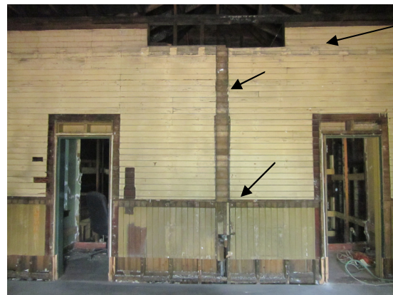
All plaster removed. Top arrow = top 2 ft. of wall covered by the lowered ceiling added in 1944. Middle arrow = The vertical shadow (unpainted area) in the center of the room, was the location of the wall separating the men's and women's waiting rooms. Bottom arrow = The shadow of the horizontal board where the wainscoting trim is missing. A scrap piece found in attic will guide reproduction of the wainscoting.
